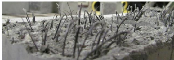
Plate 3 - Steel fibres exposed in a cut concrete section
