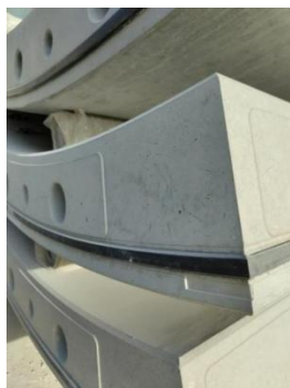
Plate 7: Steel fibres exposed on surface of tunnel linings
