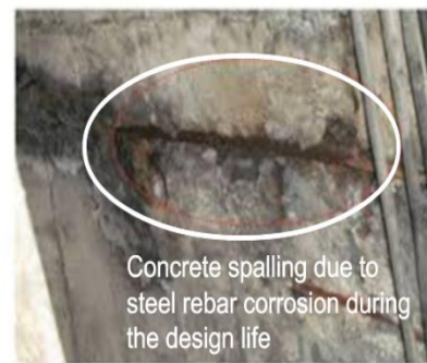
Plate 8: Concrete spalling caused by corrosion
