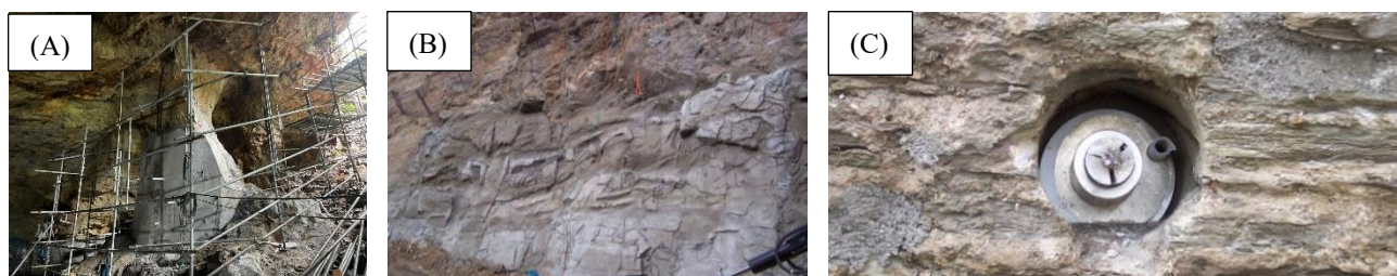
Figure 10 - (A) Rock cladding in glass fiber or aluminum with a textured and coloured finish (Lin Ma Hang, Hong Kong); (B) Completed structural shotcrete, ready for staining (Andrew et al., 2011); (C) Recessed head bolt which may be covered with facing brick or stone works.
