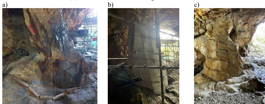
Figure 9b: Buttress B2 (Pillar P3) – (a) rock spalling as recorded during setting out the buttress extent; (b) before artificial rock cladding fixed on concrete surface; (c) after artificial rock cladding
