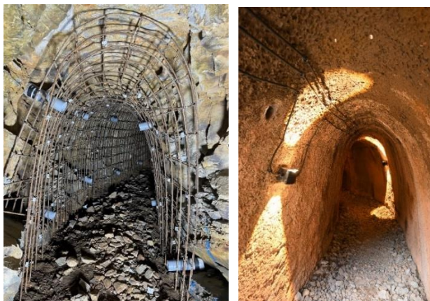
Figure 3: Paving wire mesh prior to shotcreting in Adit A6B (Left); Lighting on the shotcrete lining added after works (Right)
