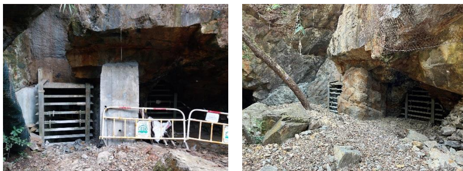
Figure 9c: Buttress B3 - (a) before artificial rock cladding fixed on concrete surface; (b) after artificial rock cladding
